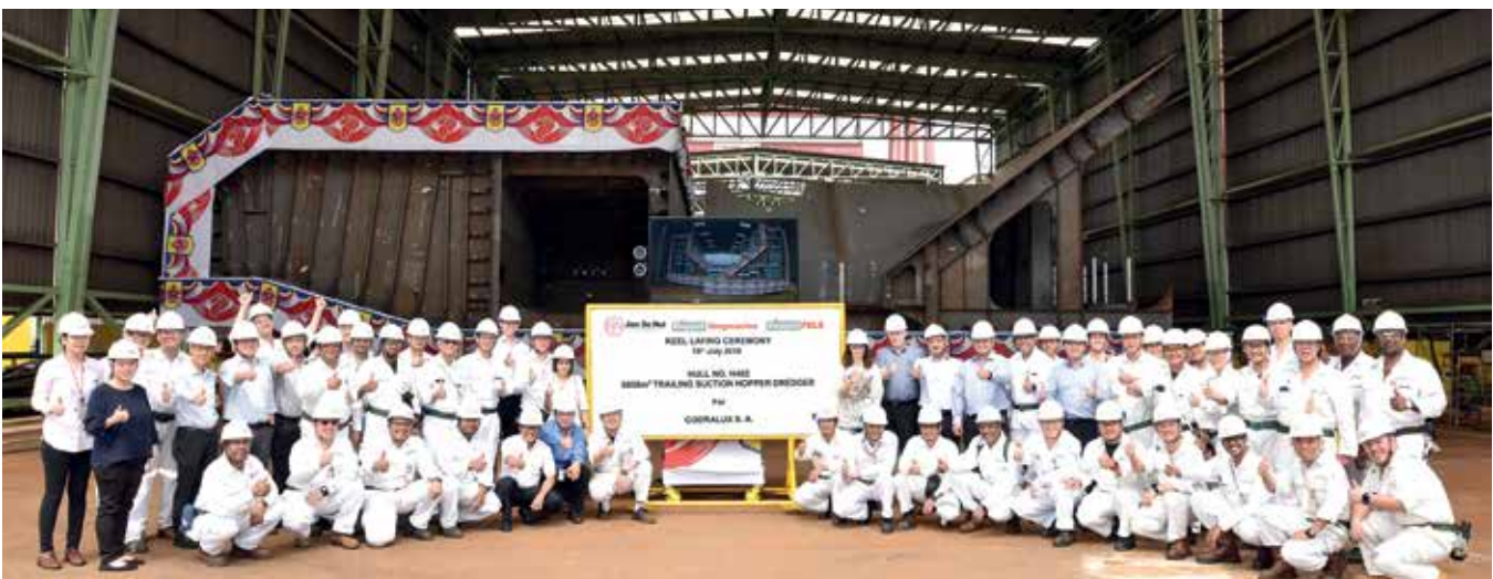
Being built in Singapore, the 6000m 3 TSHD will be the world's first EU Stage V dredger
